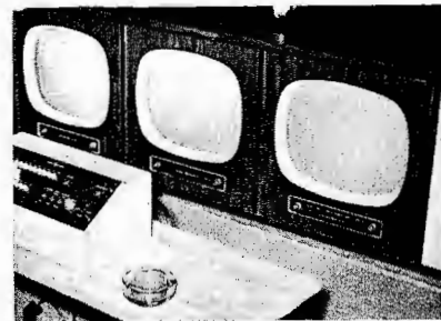
Fig. 6. CCTV video switching panel.
